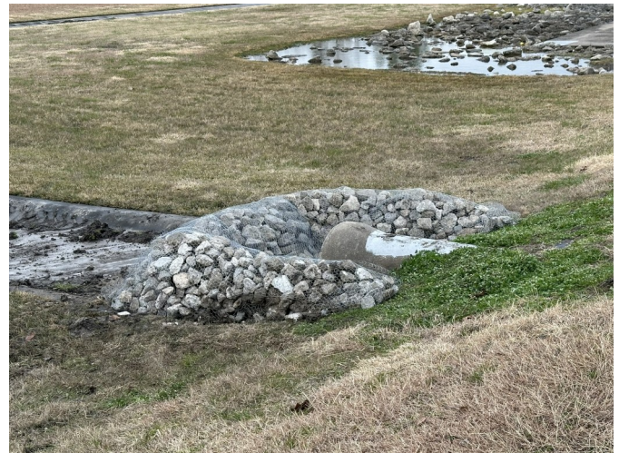
Rock Filter Dam
