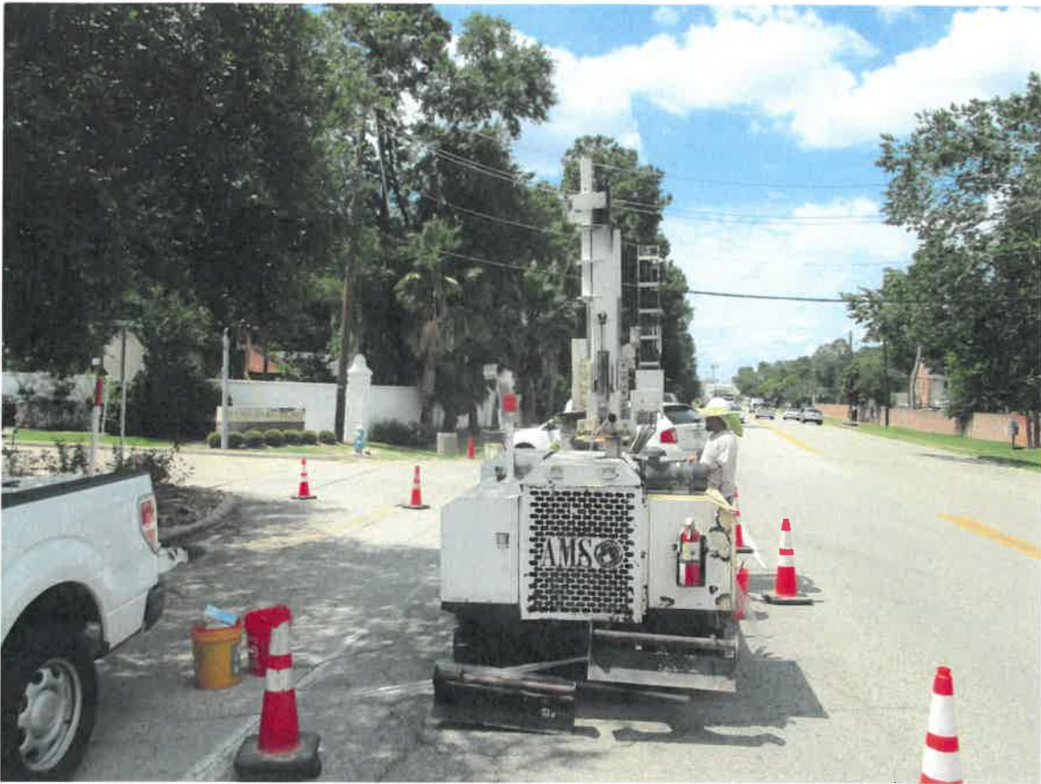
Photograph 3: View to the north of the drilling of soil boring B-22 on Memorial Drive in PPCA #5. The cross street is Boheme Drive. A former leaking gasoline station adjoined the Subject Right-of-Way to the left of the photograph.
