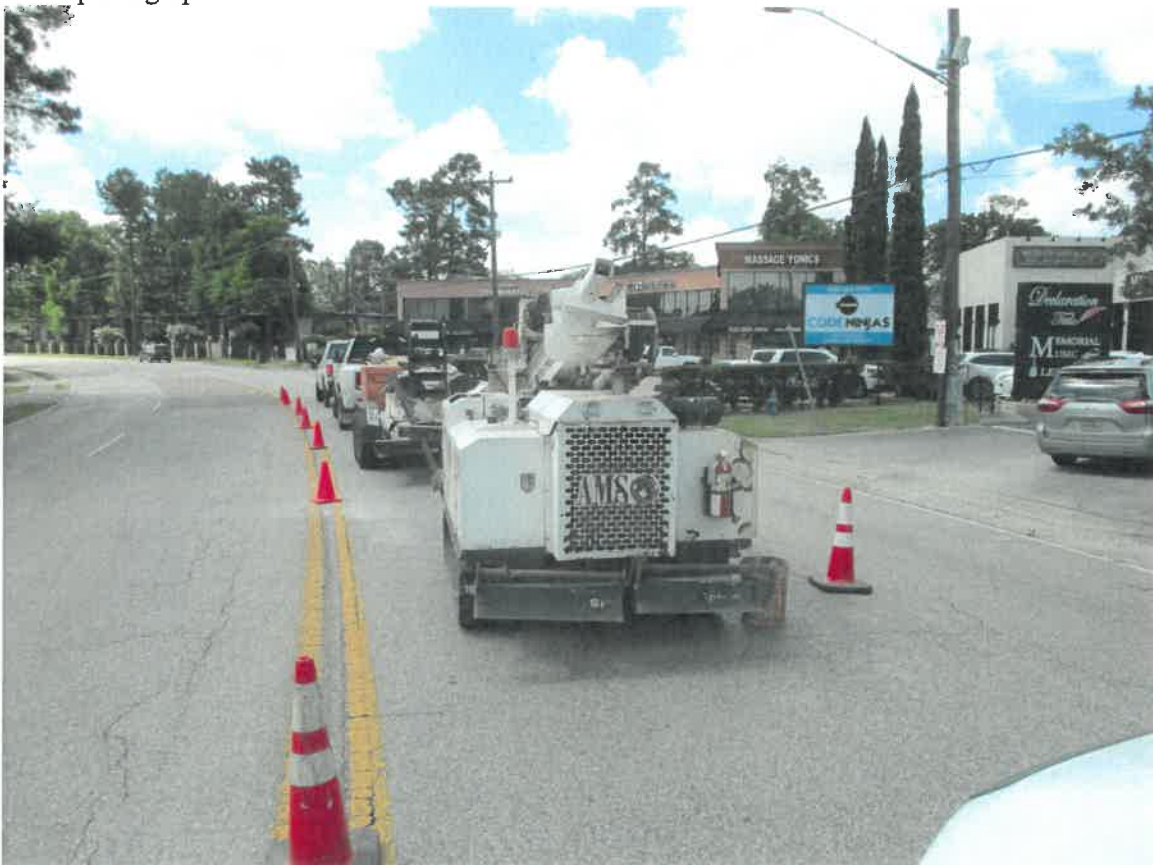
Photograph 4: View to the south of the drilling of B-24 on Memorial Drive in PPCA #5.
