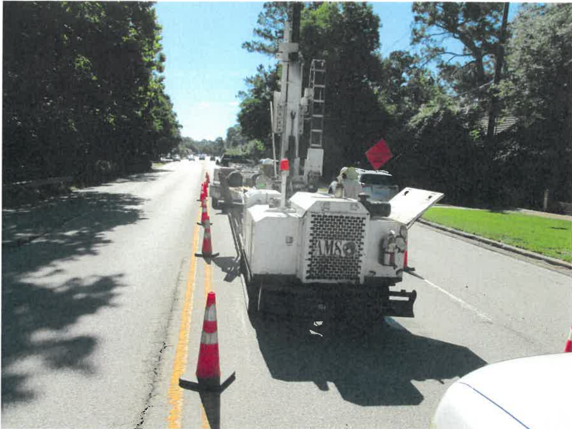
Photograph 5: View to the east of the drilling of soil boring B-26 on Memorial Drive in PPCA #6.
