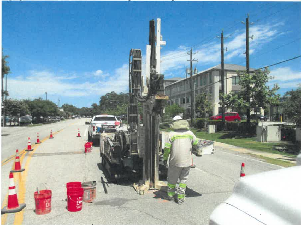
Photograph 6: View to the east of the drilling of soil boring B-29 on Memorial Drive in PPCA #6. A former leaking dry cleaners was located to the left of the tall palm tree at the left side of the photograph.
