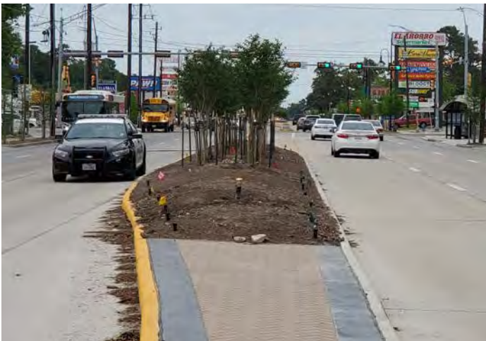
Irrigation System installed in median.
