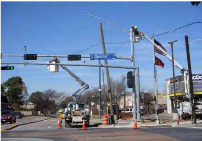
New Traffic Signal at Westview Drive
