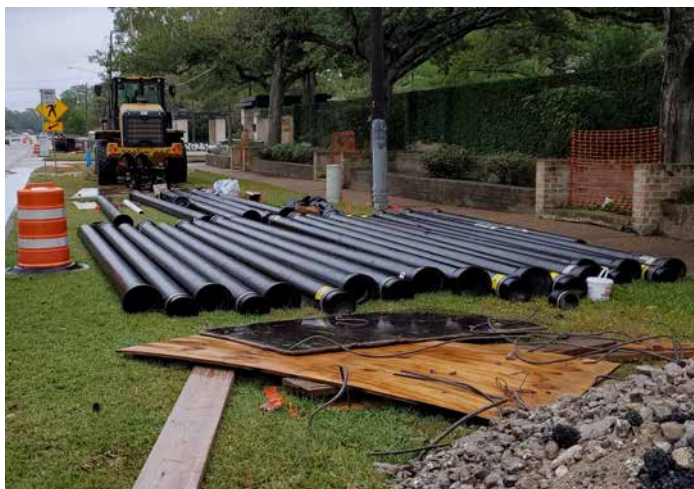
Water Line Pipes
