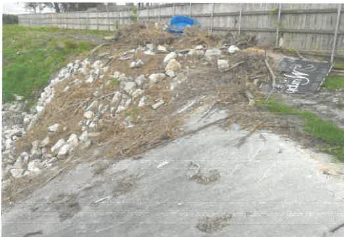
Debris cleared from west side of Bunker Hill crossing
