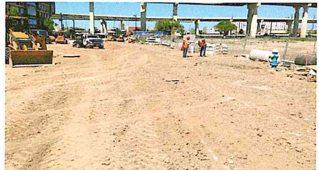
Town & Country Blvd. pavement subgrade stabilization and layout work in progress—looking north
