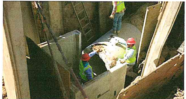
Installing 48-inch storm sewer connection between the Town & Country Blvd. and Town & Country Way storm water box culverts
