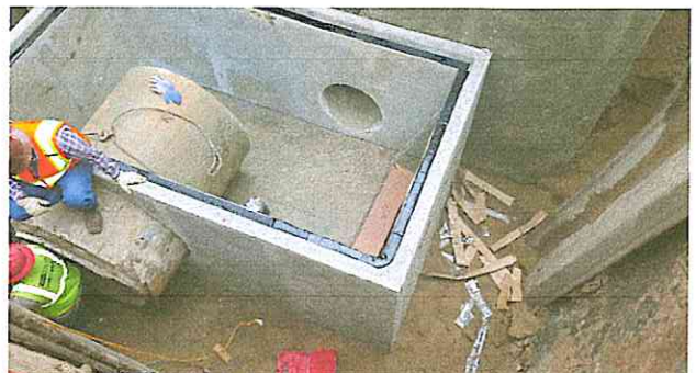
Installing storm water detention system outlet box and connection to existing storm sewer at IH10 Frontage Road
