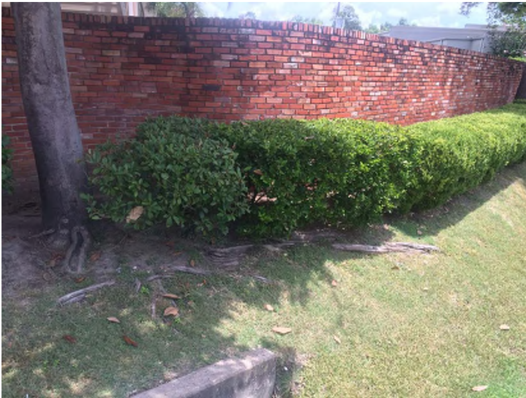
Figure 13: Roots exposed at top of bank tree no. 167.
