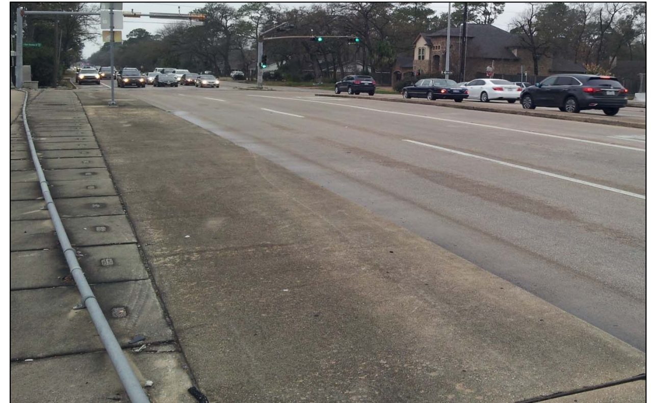
Figure 4.1: Above-ground Conduit on Memorial Drive Overpass
