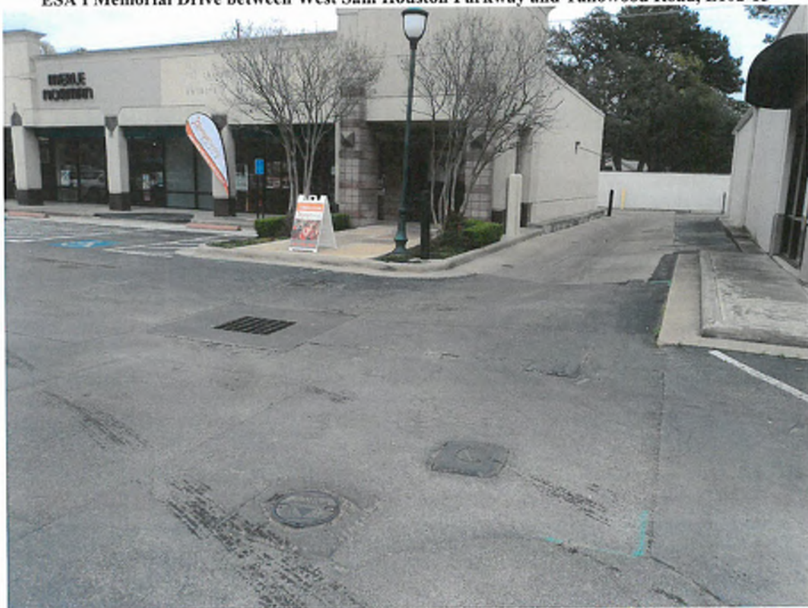
Photograph 23: View to the northeast of the former Your Valet Cleaners at 614 West Bough Lane (currently 650 West Bough Lane, Suite 100). Note the plugged monitor wells.
