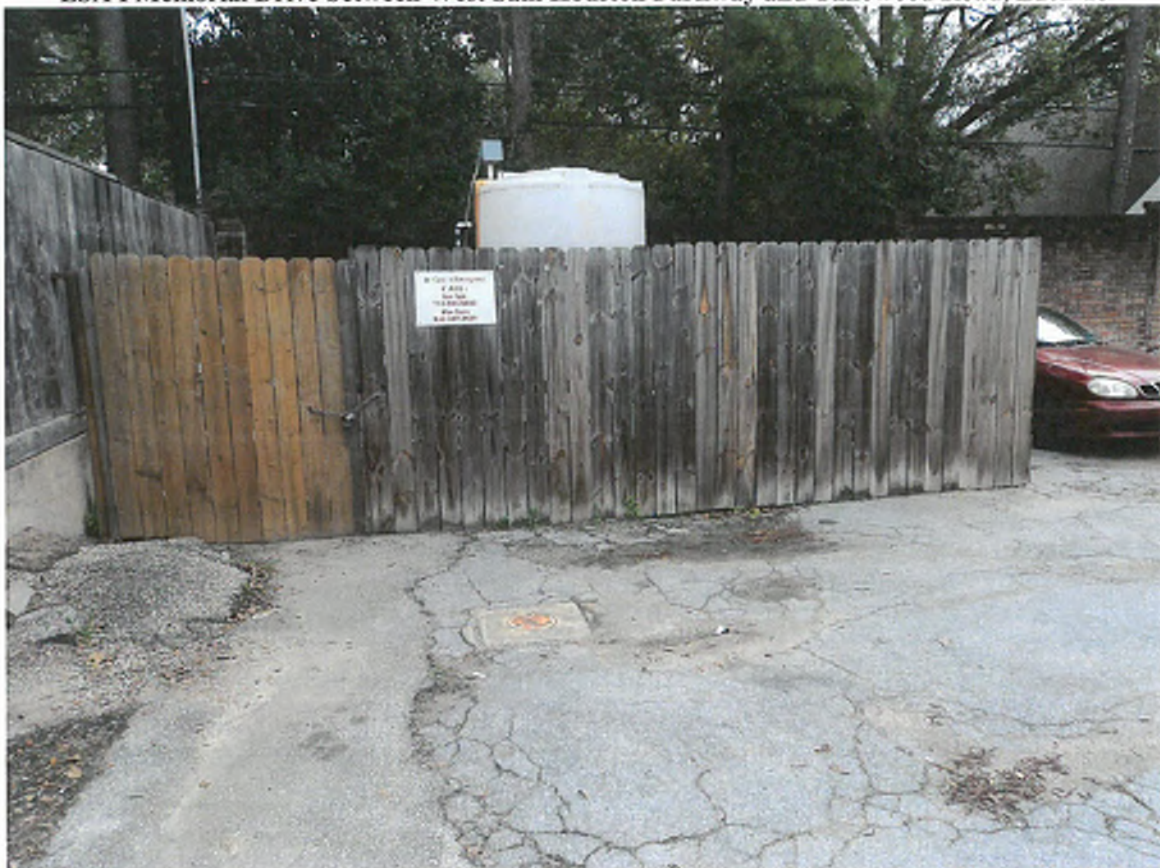
Photograph 17: View to the northeast of a monitor well and remediation system at A-1 Cleaners.
