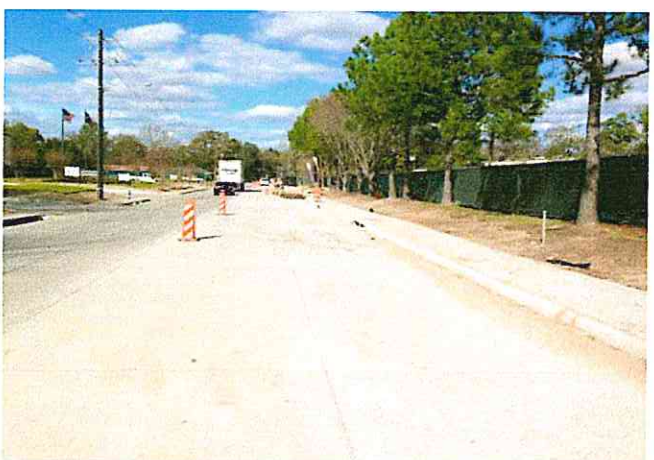
New concrete paving along east side of Lumpkin Rd., north of Westview
