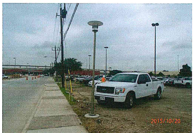
New pedestrian light Fixture
