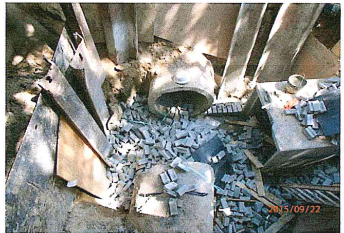
Intersection of new 4-foot by 4-foot storm box and existing 48-inch at Northbrook Dr.
