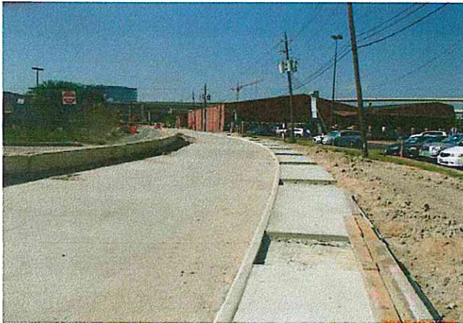
New sidewalk along west side of Lumpkin Road (leave out for brick pavers)
