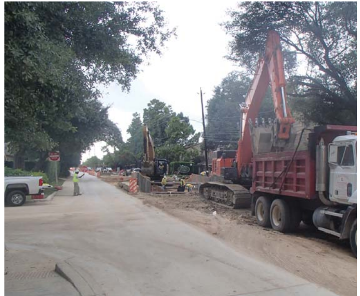
Setting new 8' x 6' storm sewer boxes in the background and excavating for boxes in the foreground near Dolphin Ct
