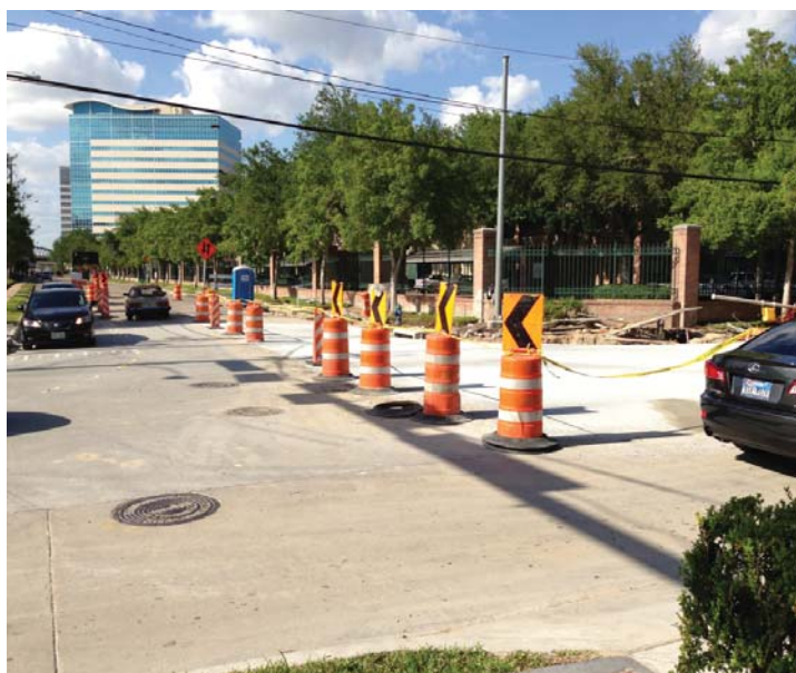
Completing the work at intersection of Barryknoll Lane and Memorial City Way.
