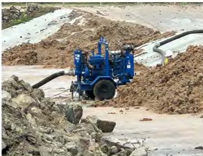
Pump for Ground Water Control
